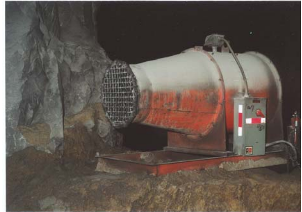
Figure 20. Axial vane auxiliary fan (note that the fan has a reducer that increases airflow momentum with a corresponding increase in entrainment and total airflow)
