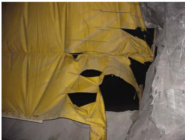
Figure 7. Typical repetitive flapping damage caused by static pressure across stopping (not blast damage)
