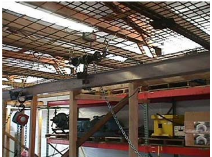
In-mine hoist system attached to wire mesh.
