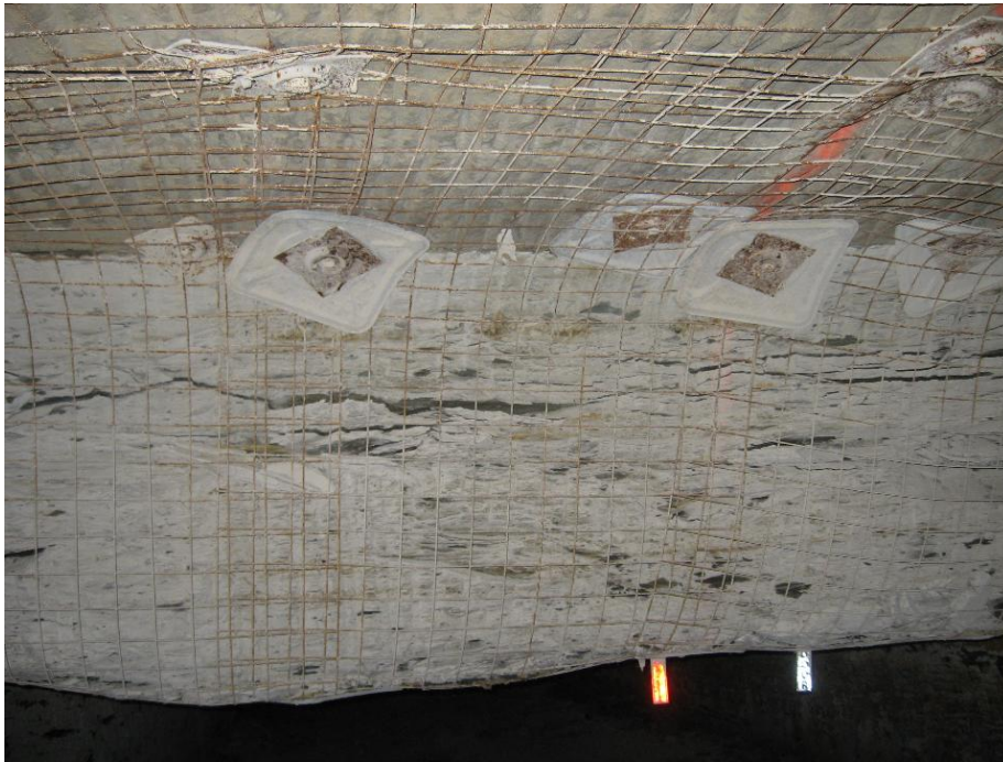
Figure 37: Bed separation in weak shale.
