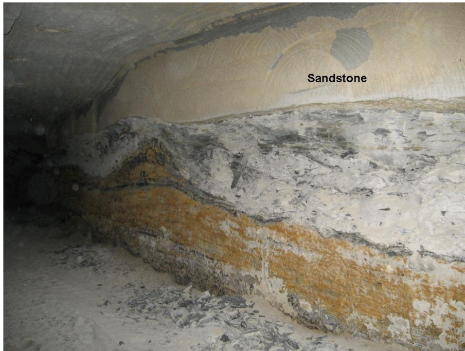
Figure 36: Sandstone layer is the roof bolt anchorage when close to the coalbed.
