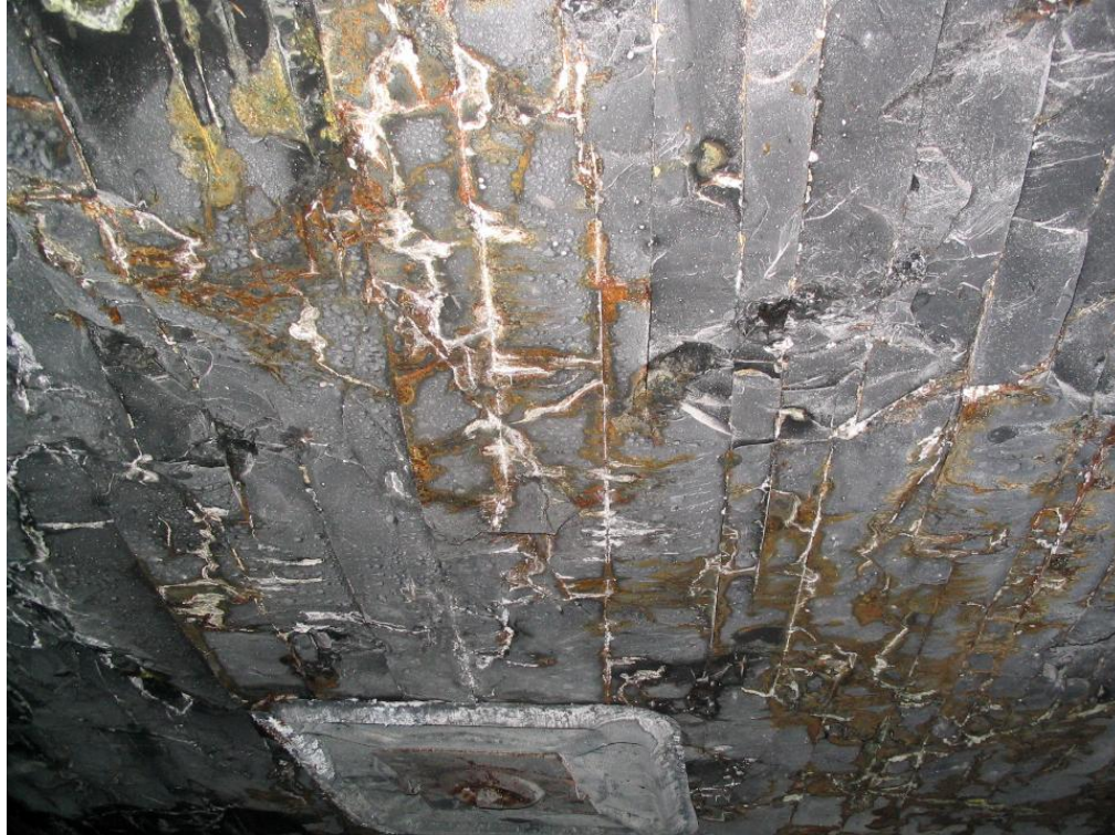
Figure 12: Joints in black shale can loosen with time causing spalling roof.
