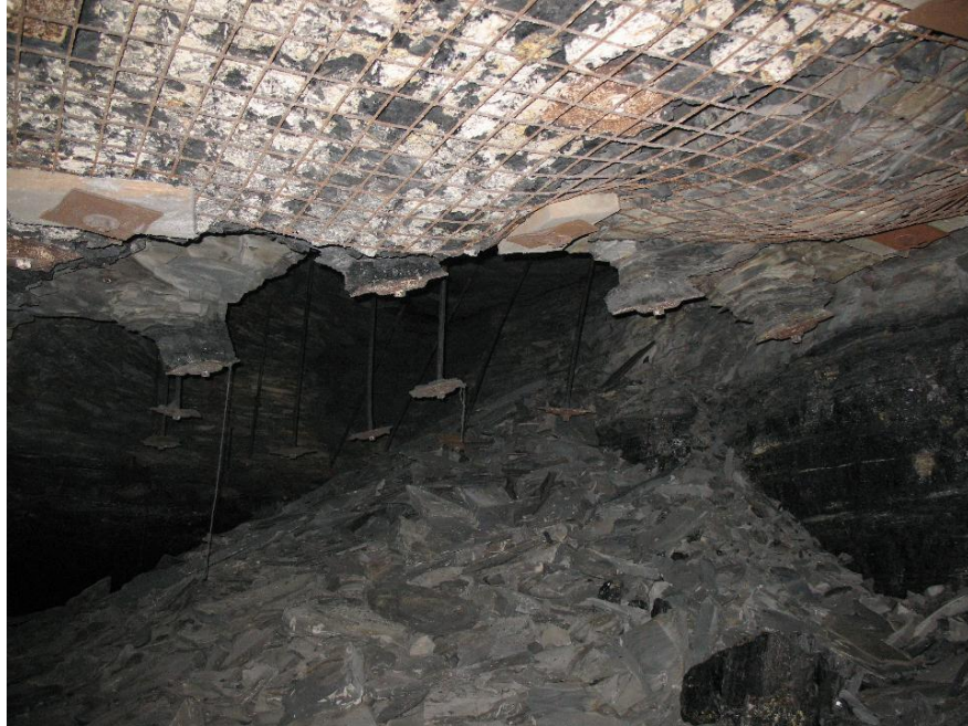
Figure 30: The screened entry is stable and the floor is clear. The unscreened entry is impassable.
