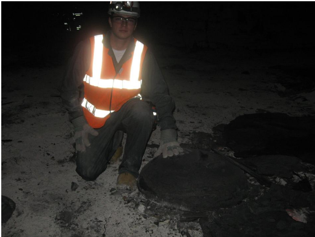
Figure 13: Siderite nodules present roof hazards.
