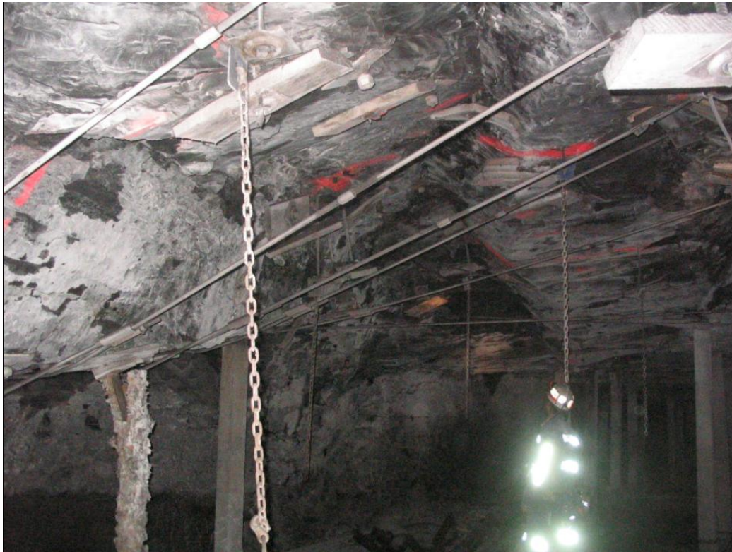
Figure 11: Slickensided failure planes cause hazardous roof conditions.
