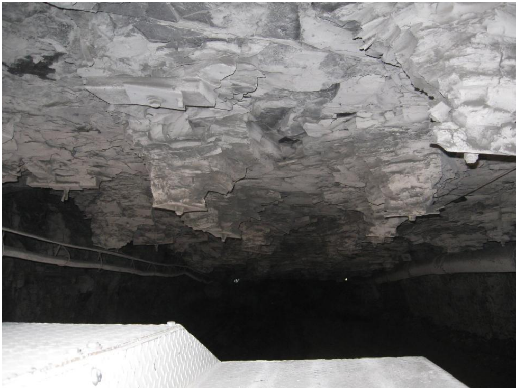
Figure 25: Deterioration of black shale exposing moisture-sensitive gray shale in a western Kentucky mine.
