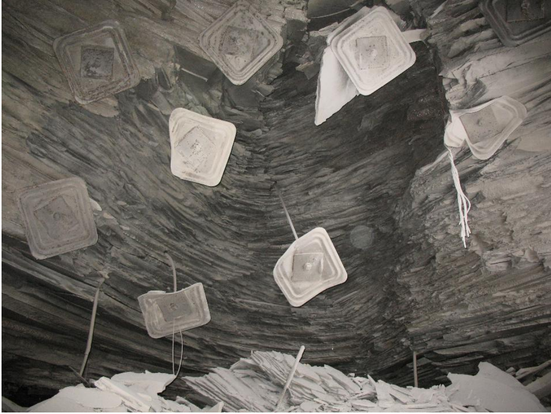
Figure 7: Roof buckling and cutter roof due to horizontal stress.
