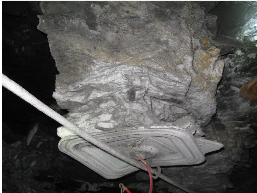
Figure 18: Exposure of moisture-sensitive gray shale leads to chandelier bolts.
