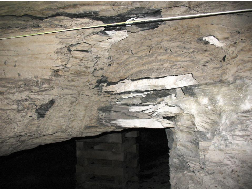
Figure 42: Stairstepping fractures extend over the pillar.
