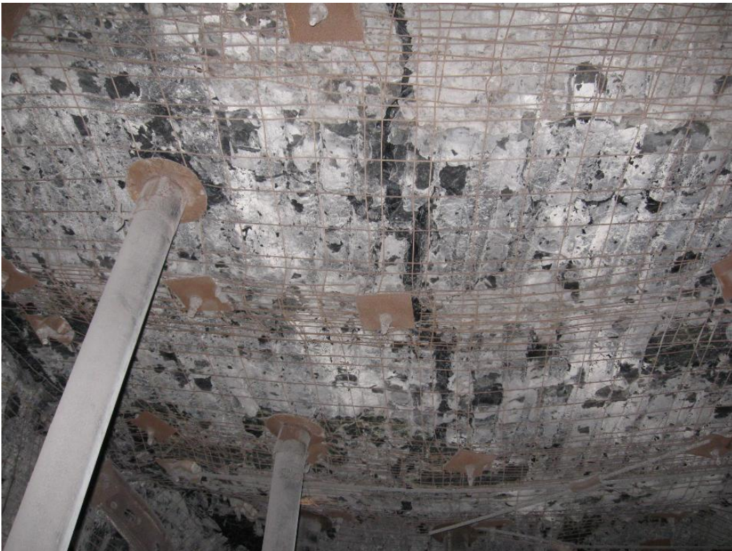
Figure 40: Tension crack in the entry center.
