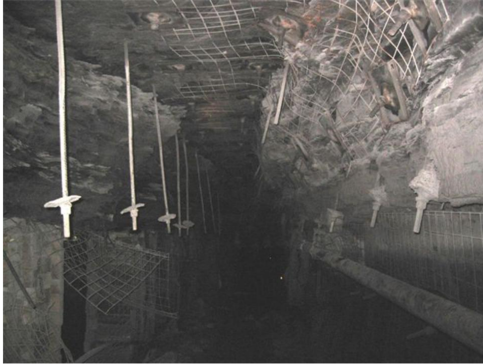
Figure 24: Rock disaggregation between bolts extends nearly to bolt anchorage.
