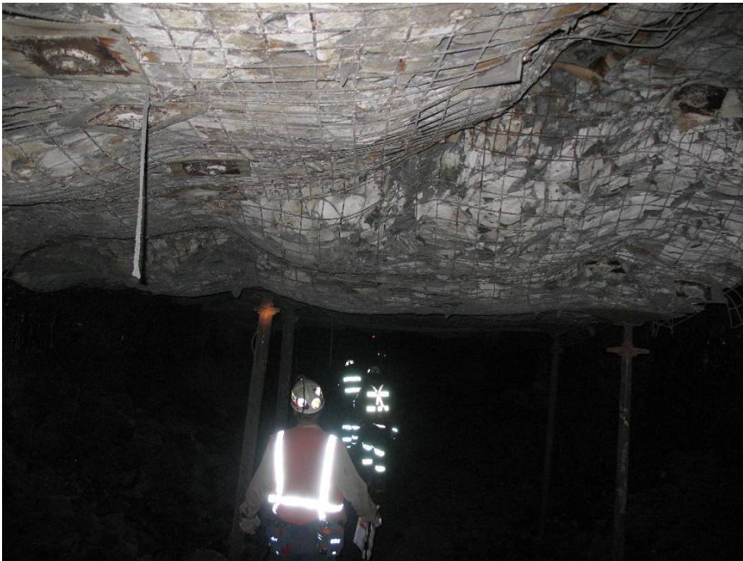
Figure 27: Roof screen holding a large amount of broken rock.
