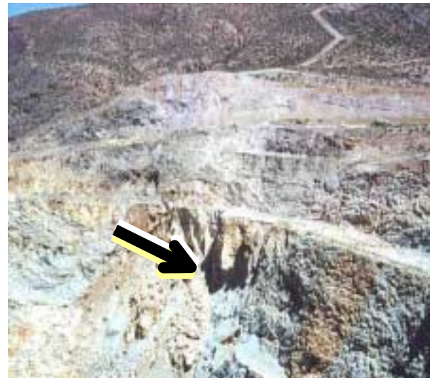
Figure 10. The overhang indicated by the arrow is a hazard to trucks traveling along the haul road because the drivers cannot see the portion of the slope that has failed below the road. The weight of the trucks on the partially failed material could cause the rest of the rock mass to fail.
