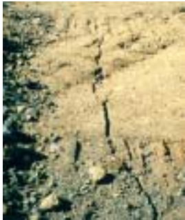
Figure 6. Example of tension cracks.
