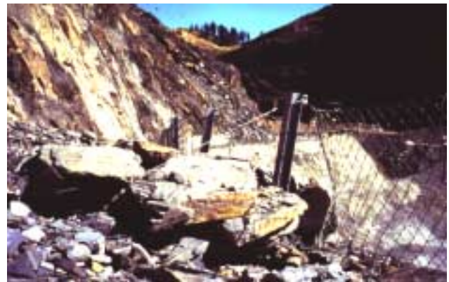
Figure 16. Catch fence installed to prevent loose rocks from traveling to the pit floor.
