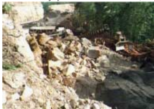
Figure 5. Fatality and loss of equipment caused by unexpected slope failure.
