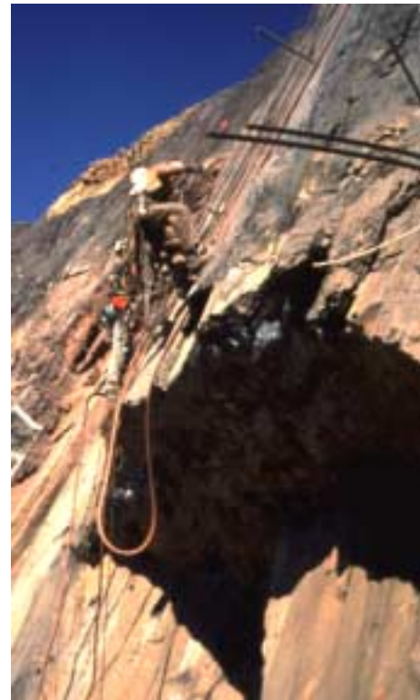
Figure 11. A worker suspended by mountain climbing gear is supporting a potentially unstable overhang with cable bolts.
