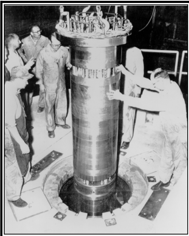
Installing reactor vessel. Idaho National Engineering and Environmental Laboratory, Idaho Falls, Idaho. Date unknown. Photo courtesy of the U.S. Department of Energy.
