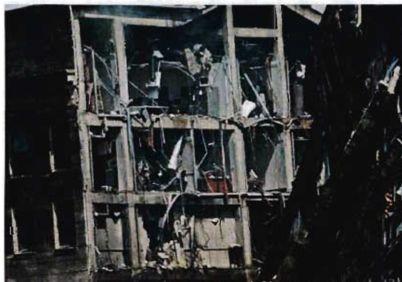
Damaged interior offices sheared open by the collapse of the E Ring.
