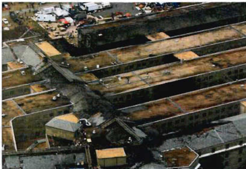
The burnt roof of the Pentagon on 14 September 2001.
