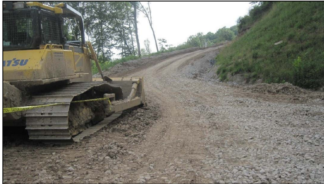
Incident scene, showing terrain and hill accessing the well site. (Photo courtesy of WV OSHA.)
