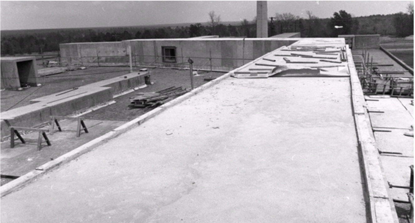
Figure E-2. Roof above the PuFF Facility in Building 235-F, April 4, 1973 (DuPont 1973c). Maintenance access and exhaust piping were installed later (DPSPF 17880-11).
