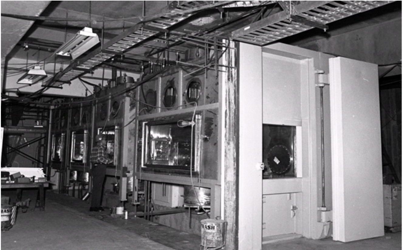
Figure E-6. Completed hot cell structure, February 26, 1975 (Du Pont ca. 1975h) (DPSPF 18813-23).
