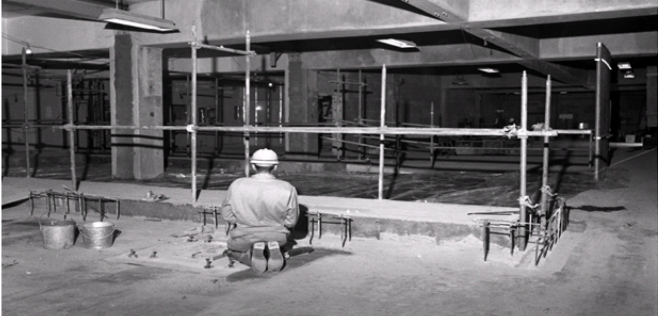
Figure E-1. Worker readying to pour concrete, April 4, 1973 (DuPont 1973b). Note that the worker does not appear to be wearing protective clothing for the prevention of radioactive contamination (DPSPF 17880-4).
