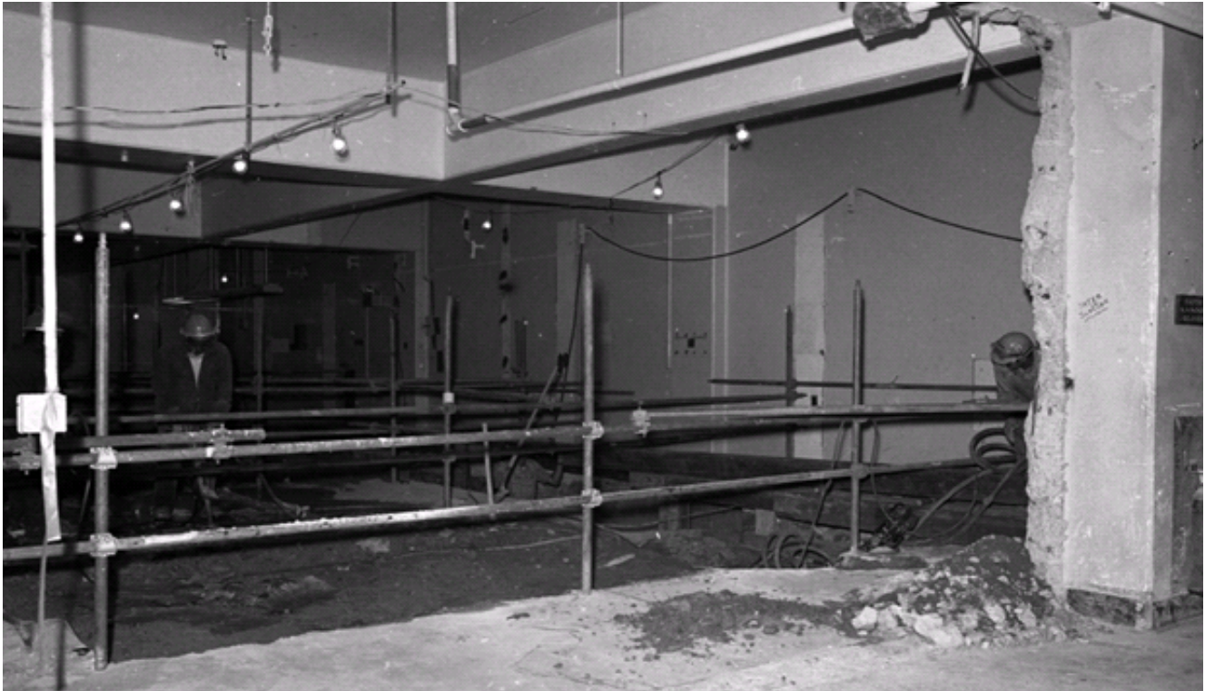
Figure E-5. Concrete removal in glovebox housing area, April 4, 1974 (DuPont 1974k) (DPSPF 17508-7).
