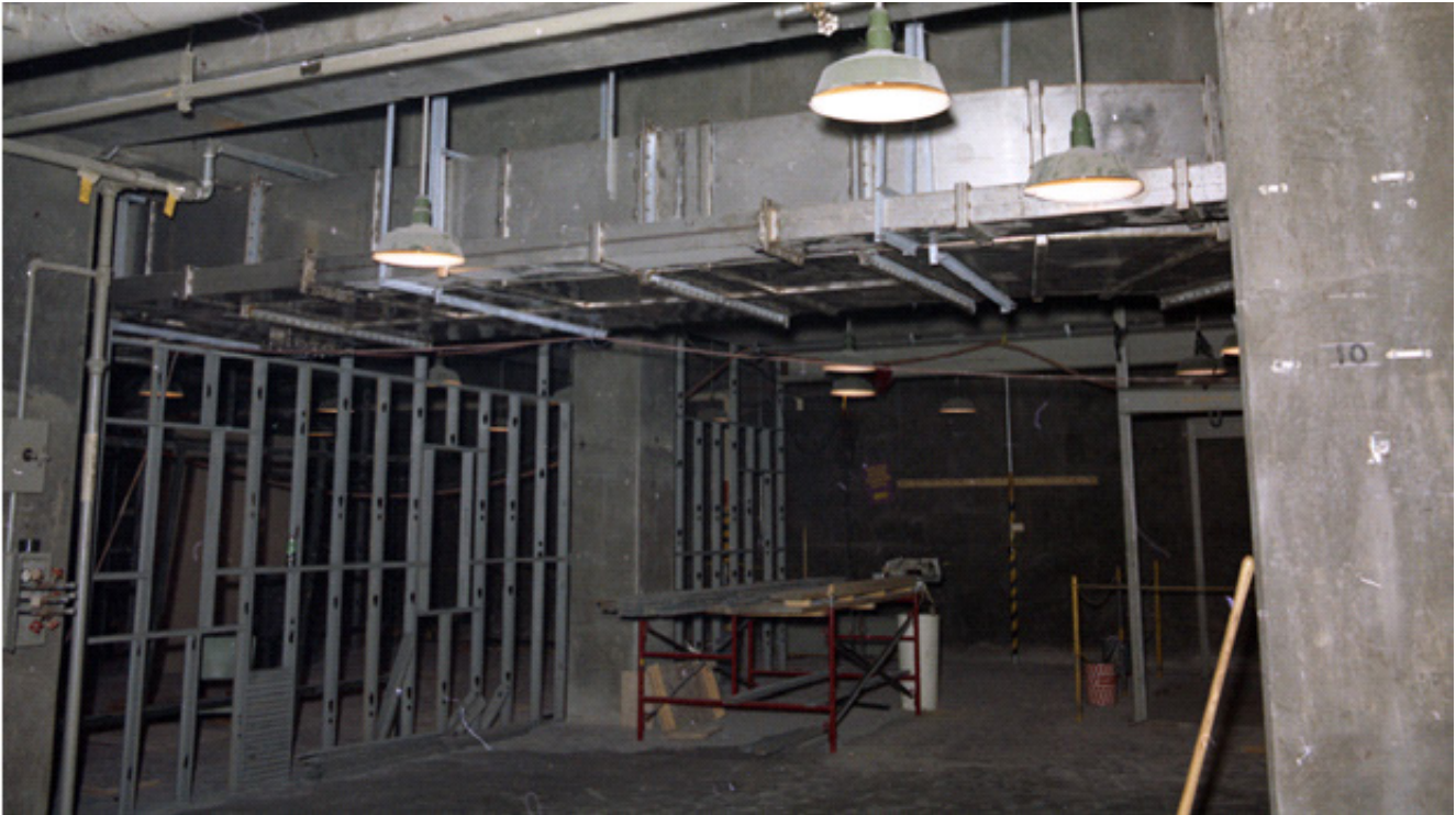
Figure E-9. Room construction, November 20, 1976 (DuPont 1976h). It is not clear what this particular room was used for. Note the clean conditions in the work area (DPSPF 18678-11).
