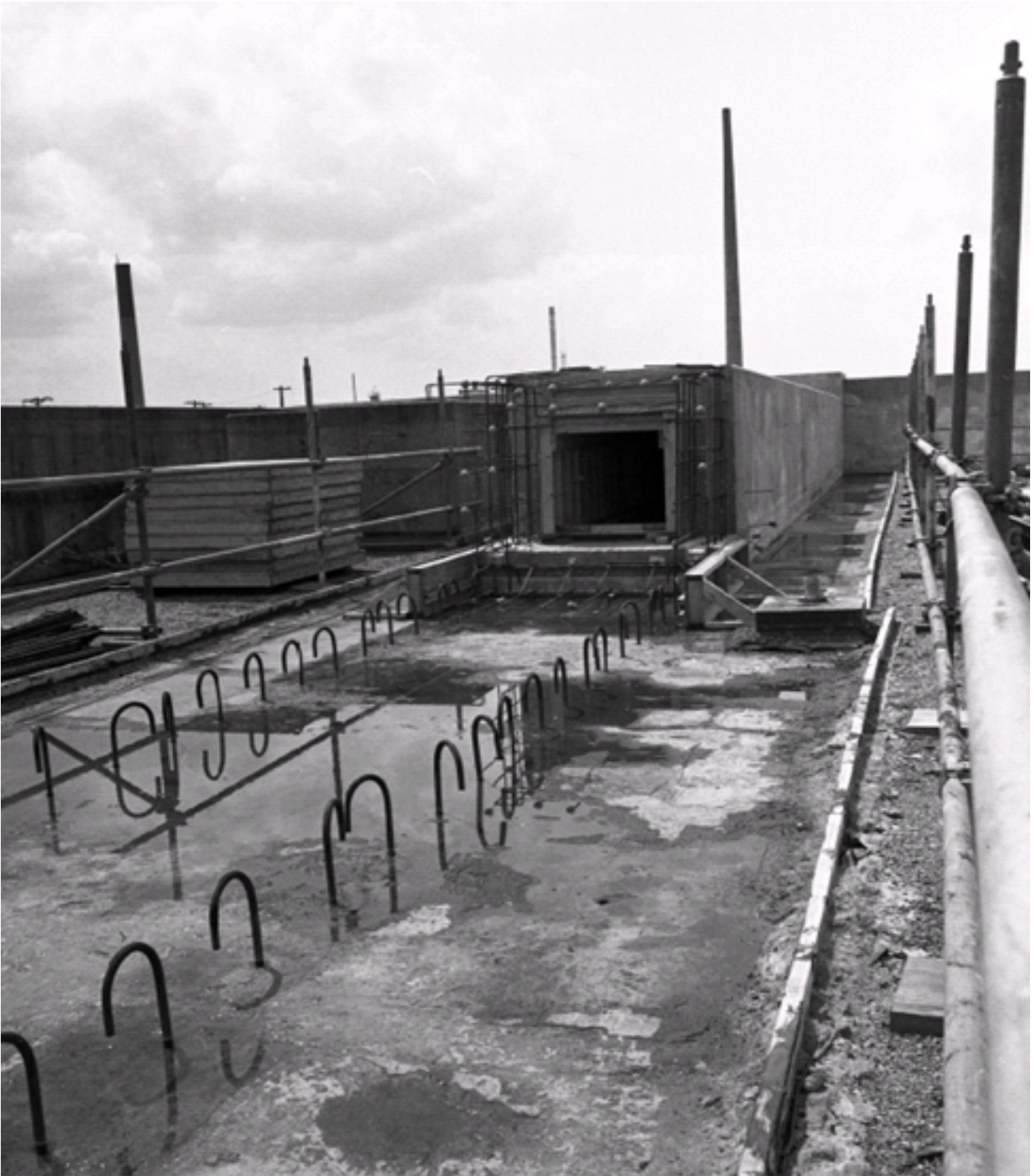
Figure E-3. Additional work on the roof of Building 235-F, April 4, 1973 (DuPont 1973d) (DPSPF 17880-12).
