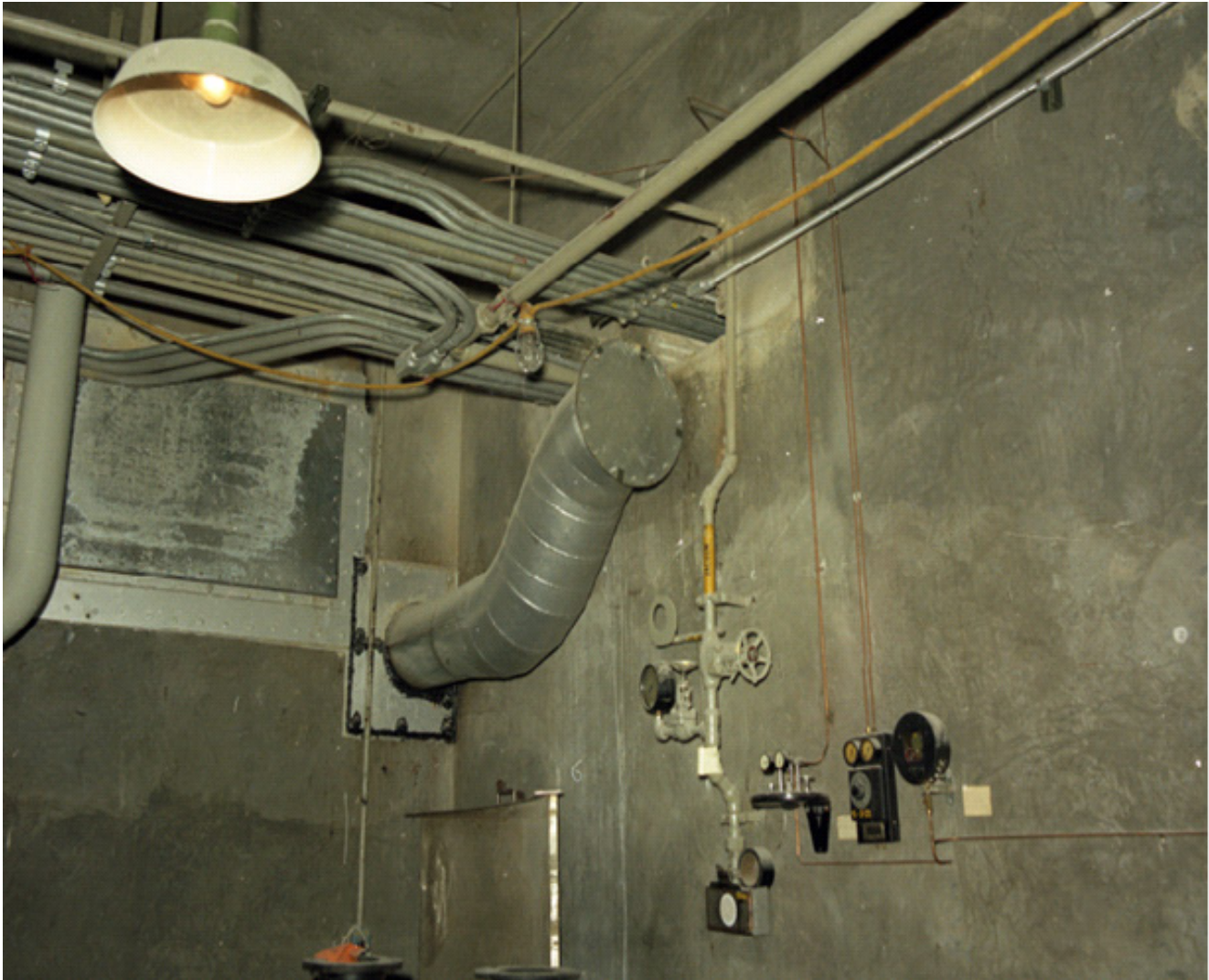
Figure E-8. Duct work in construction area, November 20, 1976 (DuPont 1976g). Note the duct to other parts of the building is closed off (DPSPF 18678-4).
