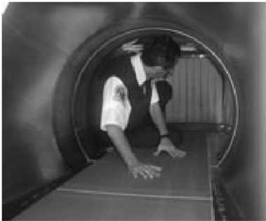
Photos 18-21: Poor work practices
